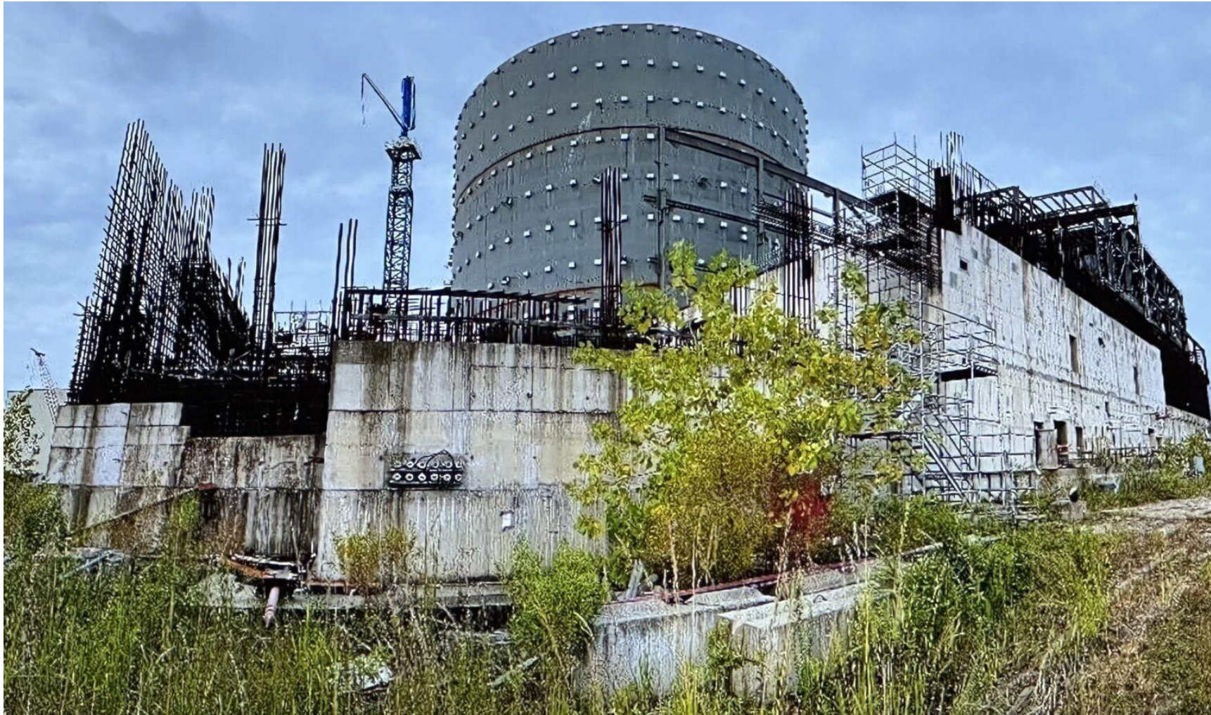
The unfinished Unit 2 nuclear reactor pictured Sept. 12, 2024, at VC Summer NPP construction site
